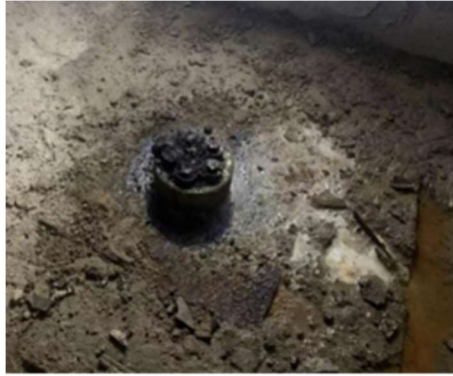
Fig.2 On-site Photograph of Anchor Rod Leakage
