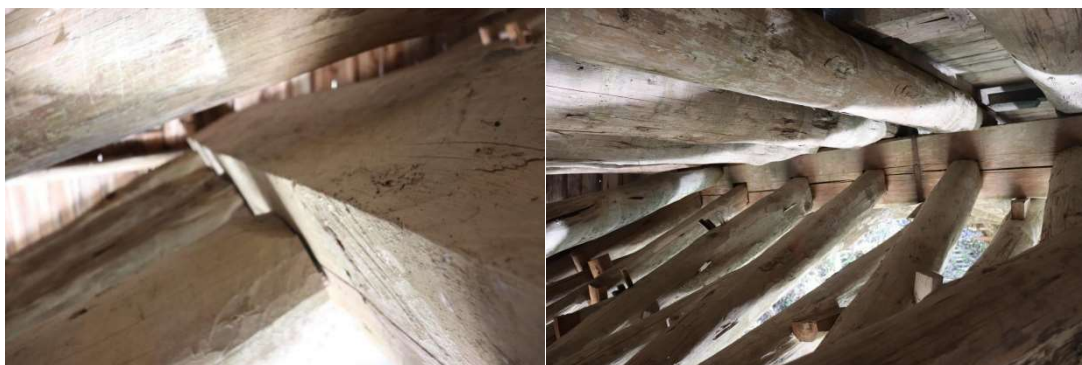
Figure 5. Left: Middle cowhead misalignment at the upper west end of a three-segment seedling; Right: Cowhead cracking on the west side of a three-segment seedling (drawn by the author)
