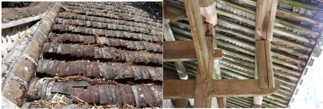
Figure 6. Left, damaged roof tiles with leaves blocking drainage; right, rotted eaves with water leaks, rafters damp and moldy (self-drawn)
